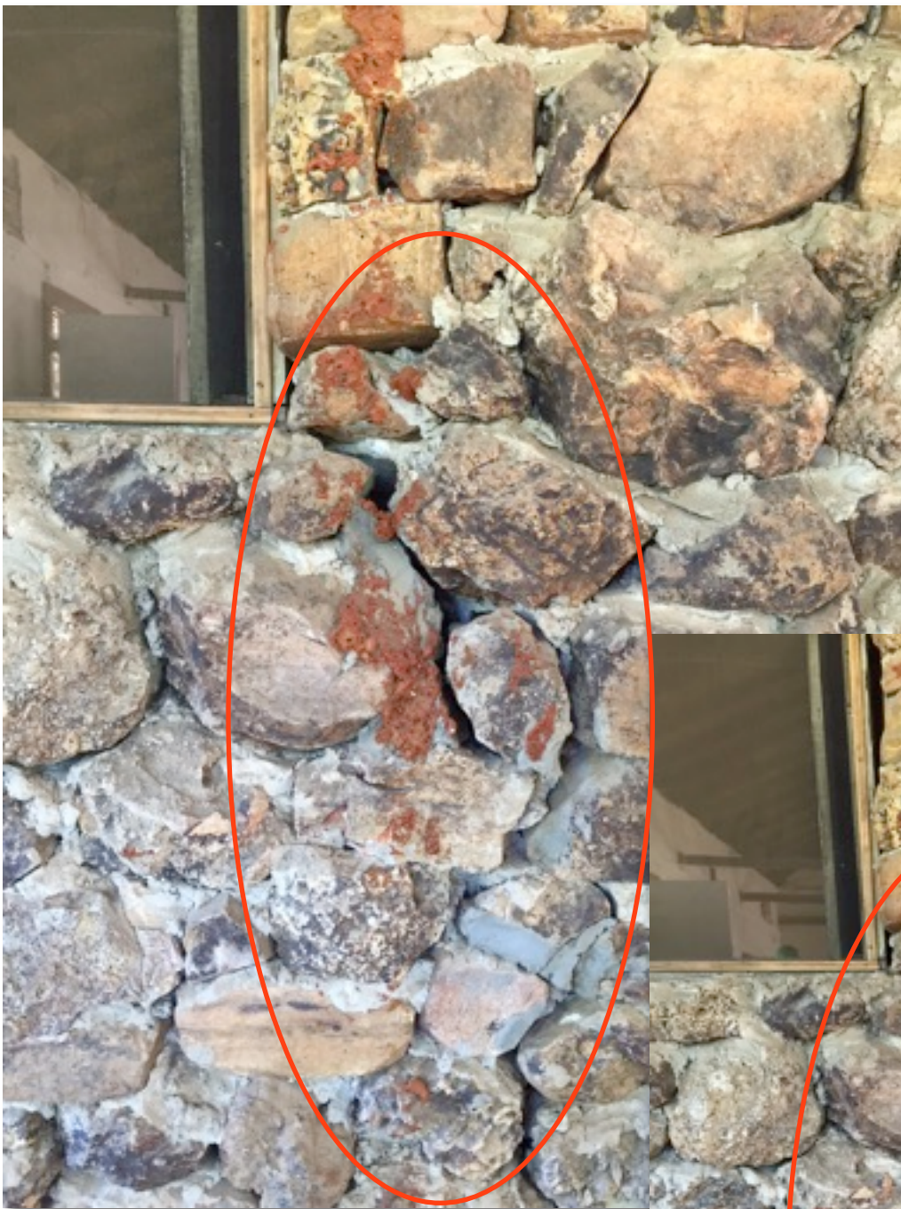
The exterior view of the open-air crack.
